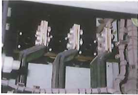
▼ Figure 4.3 Bolted connections at a busbar viewed using thermal imaging
